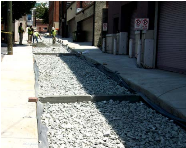
Figure 2. Concrete check dams slow water In this PICP alley in Richmond, Virginia.
