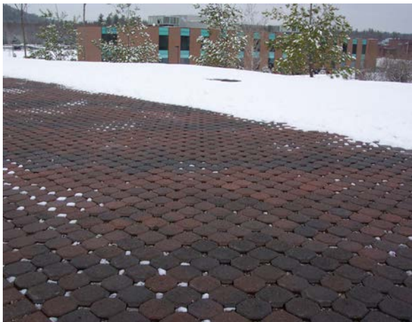
Figure 3. Snow remaining after plowing PICP can melt and reduce ice formation and slipping hazards.
