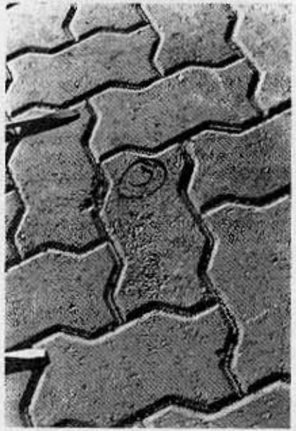
Fig. 5 - Breaking-out of aggregate particles under traffic
