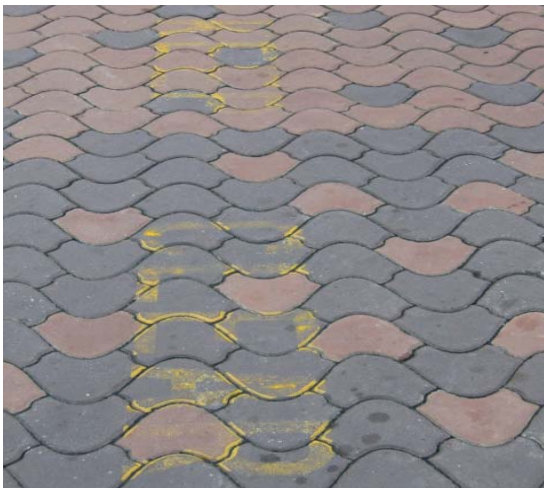
Figure 1: Faded markings on block paving
