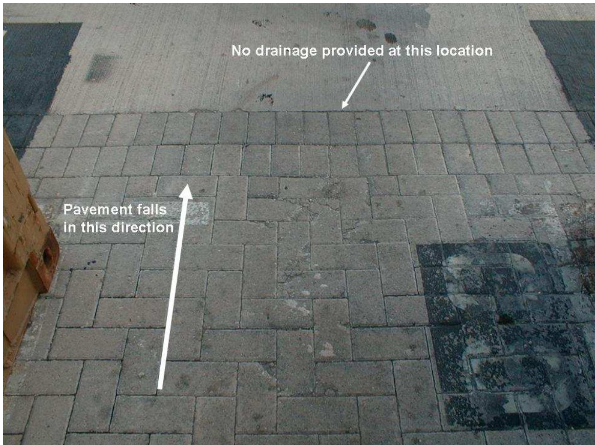
Plate 6 – Failure at Interface with Edge Restraint.
