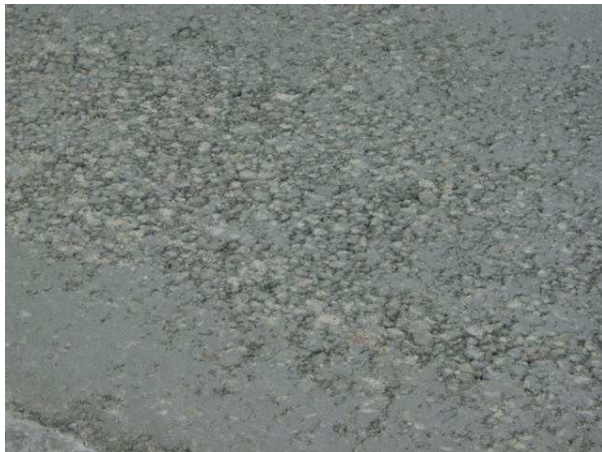
Figure 3. Segregation in finished surface of CBM.
