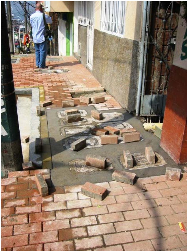
Figure 22. Many, many utility boxes.
