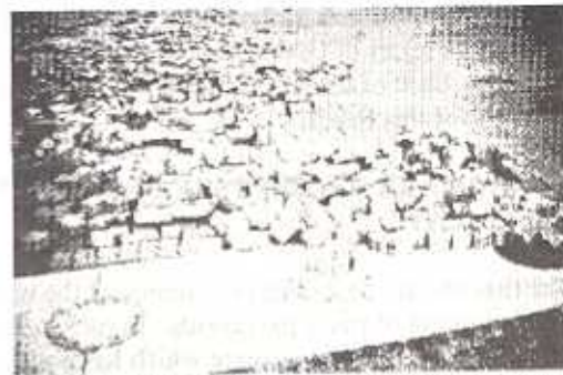
Figure 5. Jet blast has removed pavers from the Eastern Turning Circle at Luton Airport.
