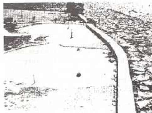
Figure 8. Pavers have been removed from a promenade at Paphos, Cyprus following a severe storm.
