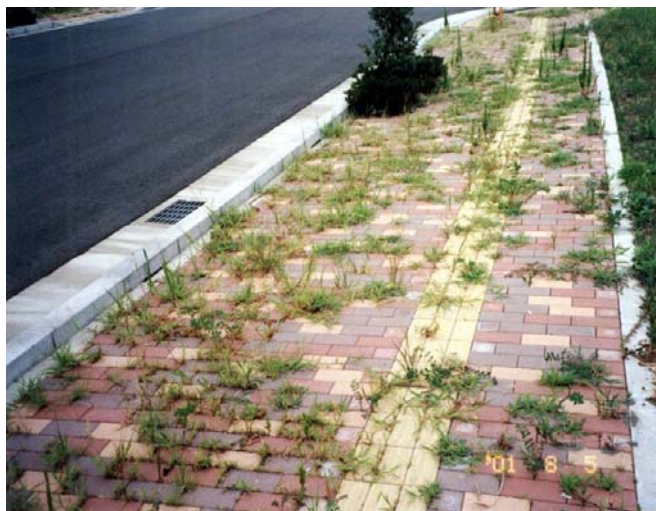
Photo 1. Weeds growing thickly on block pavement surface.
